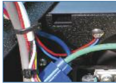
Fig 13 - Power supply and fan
